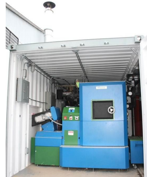
ACT Bioenergy Wood Boiler NYSAES, Geneva, NY
